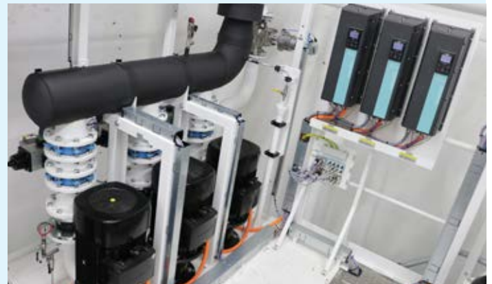
Filter pumps provide need-based, energy-saving filtration. Similarly, frequency-controlled system pumps guarantee a constant oil pressure of 5 bar.
