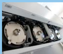
The MicroPur® filters are on the upper floor. At the moment, three filter housings are installed with two times four and one times two filter housings.
