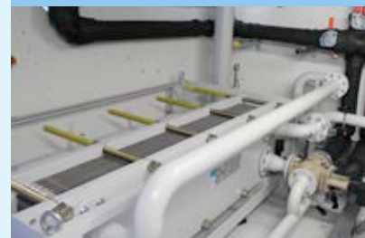
The heat exchanger keeps the temperature of the grinding oil at a constant 24 °C.
