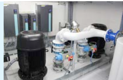
Redundancy reigns, in other places among the large 55 kW supply pumps.
