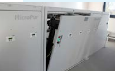
For its new tool grinding shop, HAIMER invested in a central cooling lubricant system from KNOLL; its core element is the MicroPur® superfine filter.
