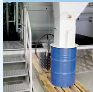
The metal carbide swarf is discharged via a scraper belt conveyor to a disposal drum, where they sediment under their own weight. The residual oil above is aspirated and returned to the circuit.
