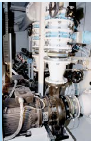
The process and filter pumps employed for this purpose conform to the new efficiency class IE3.
