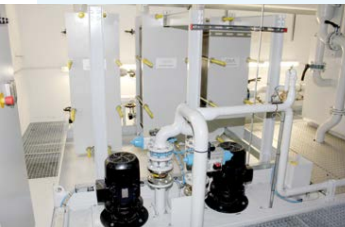
The required constant temperature is guaranteed by three plate heat exchangers, each with a capacity of 135 kW (image background).
