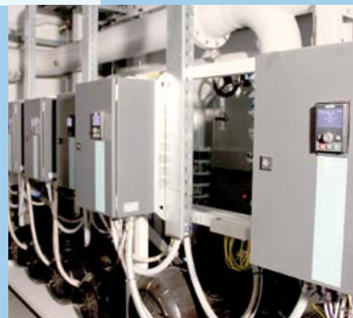
All important pumps are equipped with a frequency inverter, thereby contributing to energy-efficient system operation.
