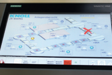
A Siemens PLC controls the KNOLL assembly and transport system. The monitor displays the system layout.
