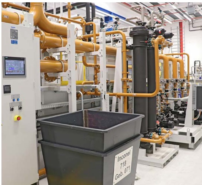
An important component of the new production system at MTU - the cooling lubricant central system that KNOLL delivered, which is responsible for cleaning, tempering, and refilling the medium.
