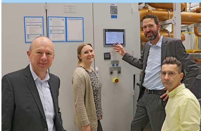
KNOLL project manager Lothar Schmid explains special functions on the control cabinet display; in the middle, Christina Braun and on the right, Zeljko Leovac (both MTU); on the left at the front, KNOLL regional sales manager Gerhard Fink.
