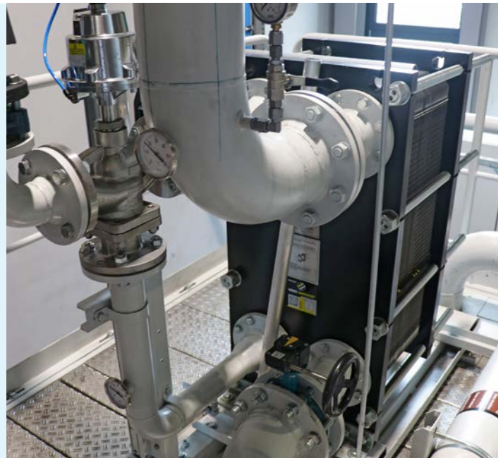
A plate heat exchanger keeps the cooling lubricant at a constant temperature.
