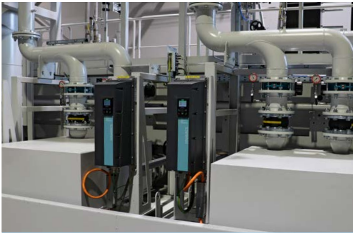
The two dirty water outflows for the filter modules can be seen to the left in the back of the picture. On the right are the two clean medium outflows, which supply the machines with clean medium redundantly.
